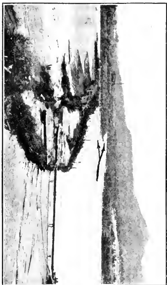
FIG. 5.—HYDRAULIC-FILL DAM, HANLON HEADING, FROM ARIZONA SHORE TOWARD ALAMO INTAKE CANAL, AUGUST 29TH, 1915.
